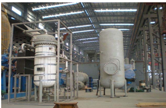
Vessel compressor unit is being assembled at the workshop of Shenghui Gas Chemical Systems, in which aims at being a advanced Cargo System provider not only a Cargo Tank fabricator.
